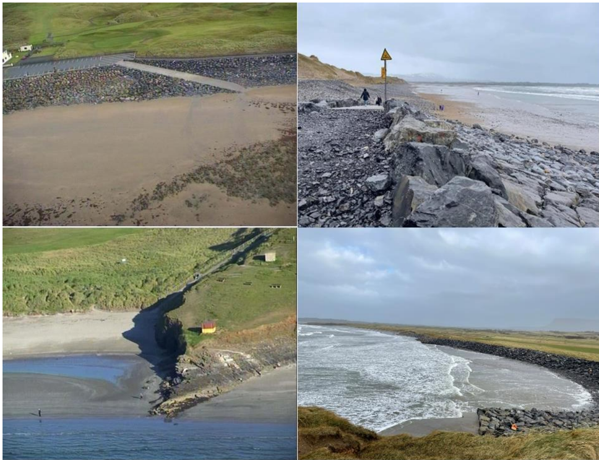
Figure 3: Top left: Oblique imagery (2003) of rock armouring and beach access ramp at Strandhill at low-tide, Top right: Present rock armouring and access ramp at Strandhill, Bottom left: Oblique imagery (2003) of unarmoured Bromore point at Rosses Point and Bot
